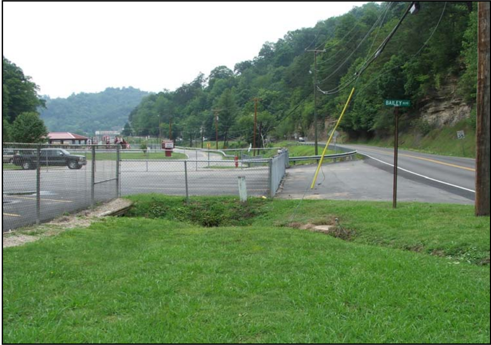
KY 1460 at Bailey Blvd near Pikeville Elementary. Chloe Creek passes under the roadway at this location; local reports indicate water pools in roadway at times.
