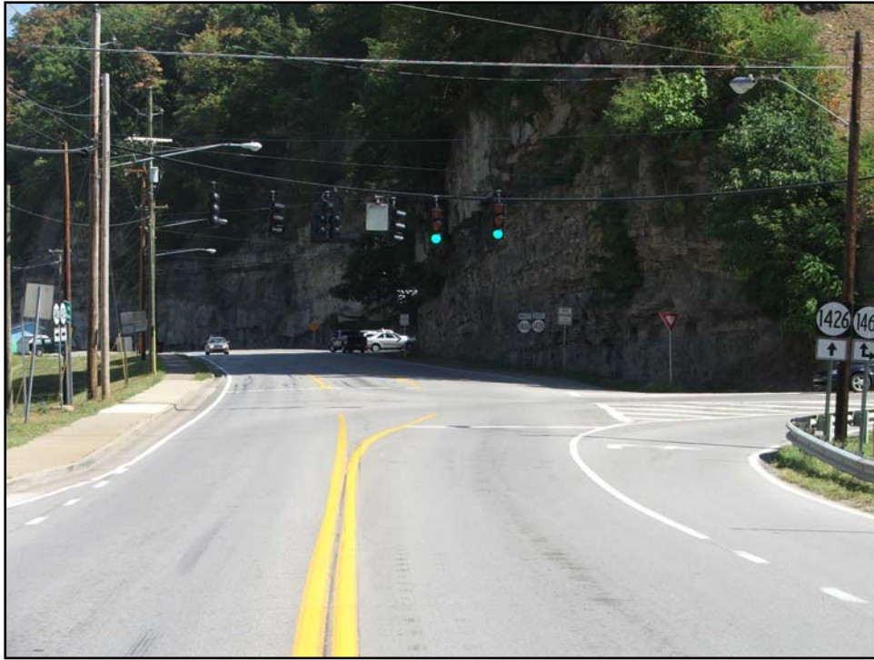
Rockfall area east of KY 1426
