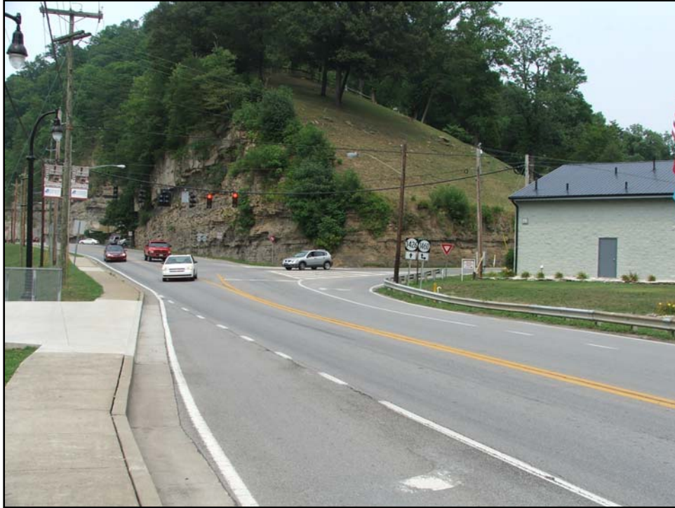
Cut slope at KY 1426/KY 1460 intersection with rockfall hazard. Dils Cemetery sits atop ridge
